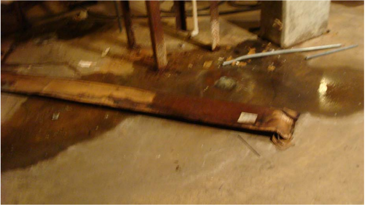
Figure 5 – Water in Building 128H Mechanical Room which poses a mold problem
