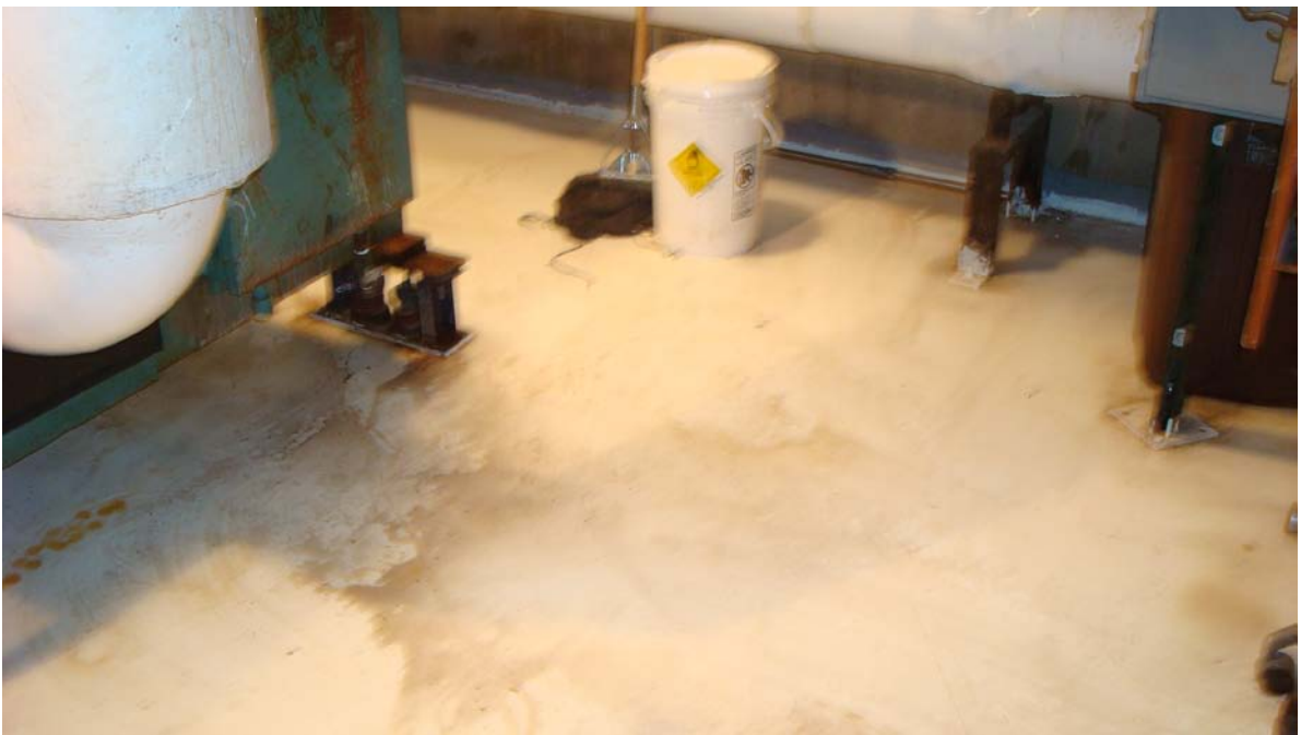
Figure 4 – Water on floor from leaking HVAC unit in Penthouse in Building 130H
