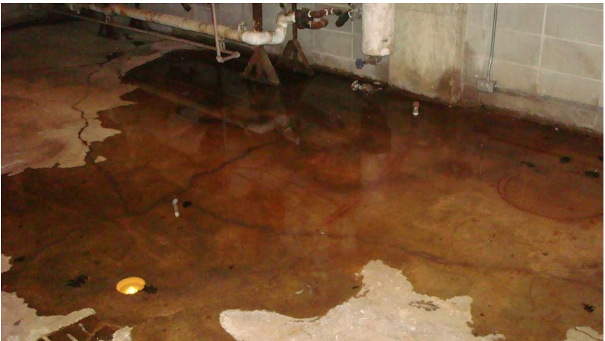
Figure 6 – Water in Building 129H Mechanical Room which poses a mold problem
