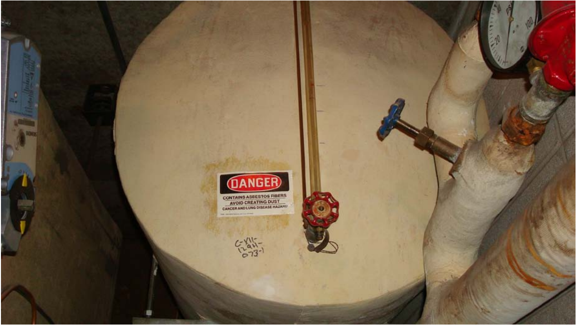
Figure 7 - Bldg 128H Asbestos in Fan Room
