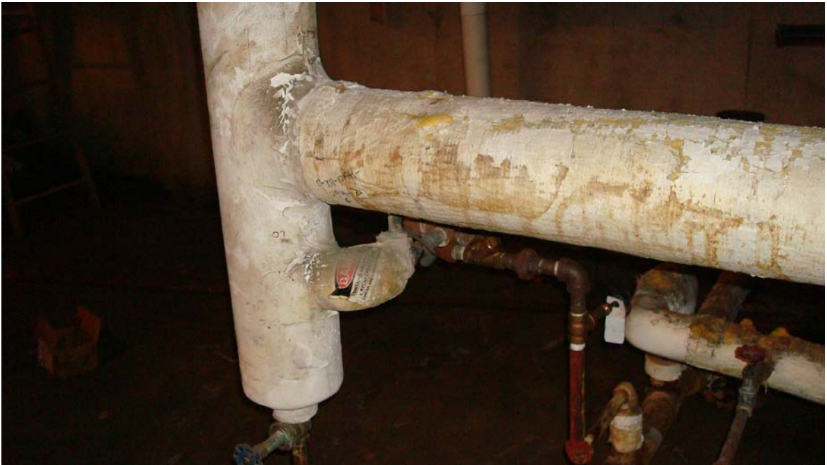
Figure 8 - Building 129H Asbestos fittings in Mechanical Room
